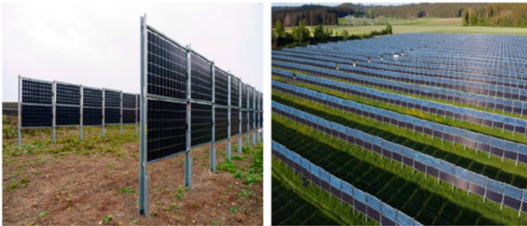
Figure 3.C.2.b-5. Vertical Solar PV Arrays 45
