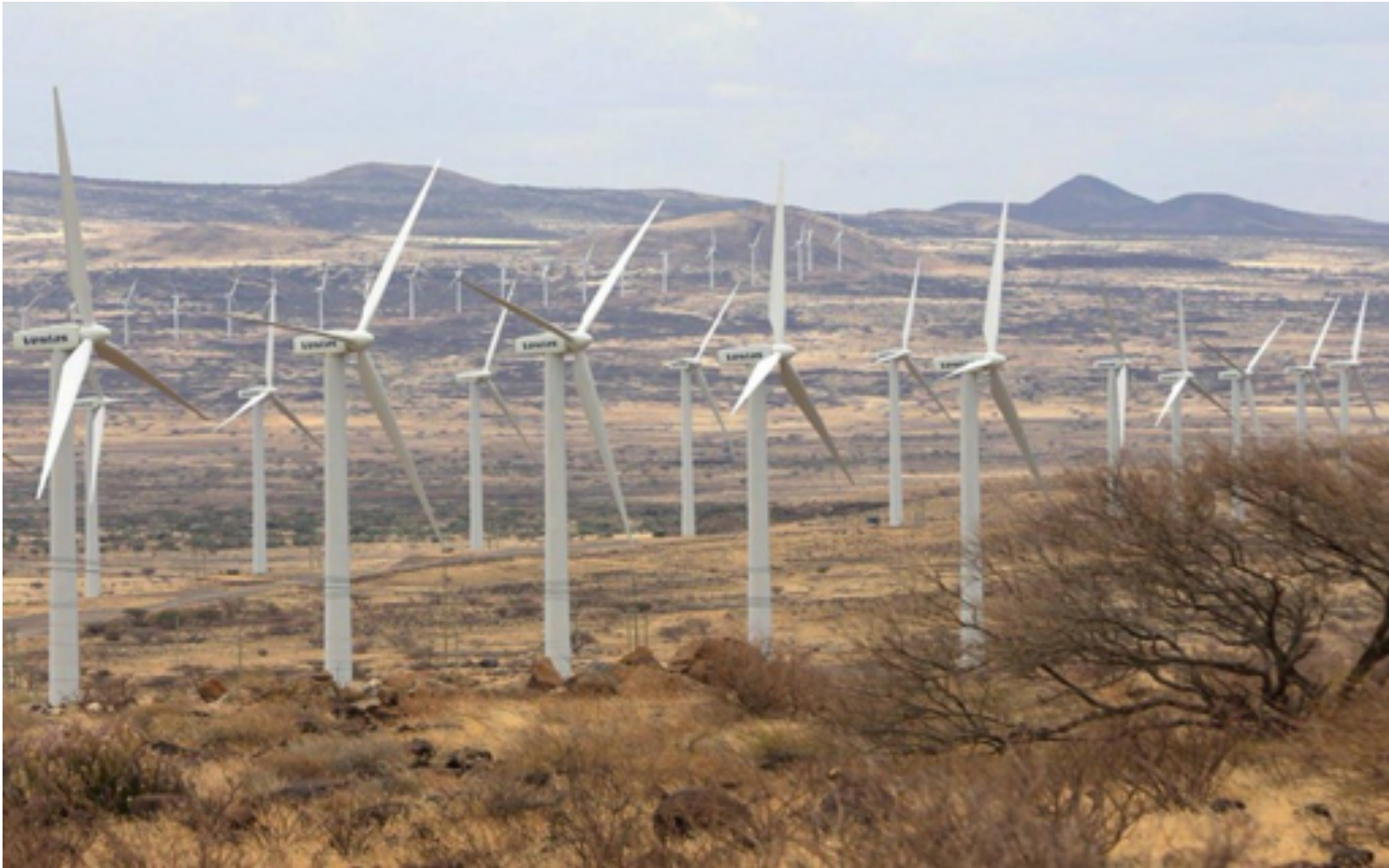
Lake Turkana Wind Farm, Kenya KENYA ELECTRICITY TRANSMISSION CO.
