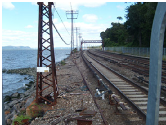
Railroad tracks that run only a few feet above the Hudson River illustrate the vulnerability to climate change and sea level rise of infrastructure located near water bodies. Tidal as far north as Troy, the Hudson will directly experience higher ocean levels and storm surges.
