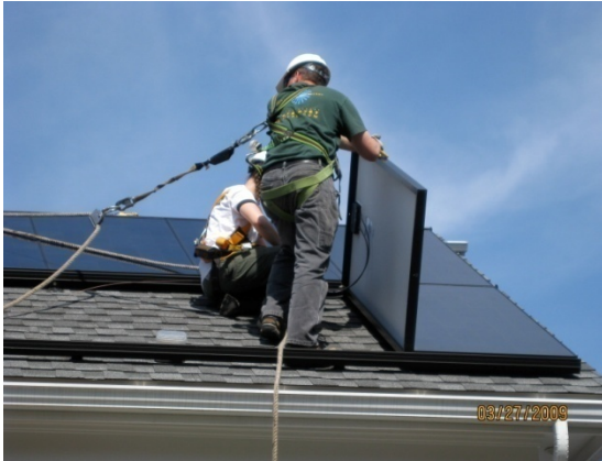
Solar panels on the Town Hall roof in the Climate Smart Community of Red Hook are reducing power bills so successfully that the town has applied to expand the installation and develop renewable energy improvement projects for other local government facilities. (Photo courtesy of Town of Red Hook)
