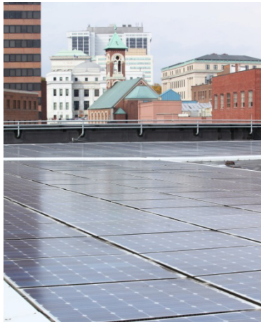
Rooftop solar panels provide renewable power for many buildings across New York State. Here, the array on the Dormitory Authority's Albany headquarters. (Photo courtesy of DASNY)
