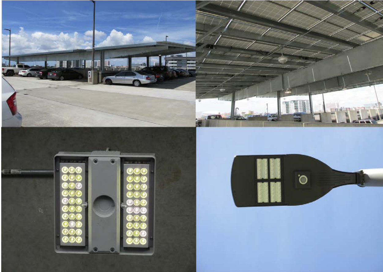
Figure 1-2. USFSP Parking Garage PV System and LED Fixtures
